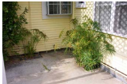
Figure 2. Cyperus (wrong plant) in foundation crawl space accesses (wrong location).
